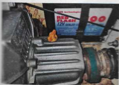
Red Flash 1100 AGM battery alongside the gearbox in the engine room
