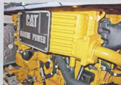
ABOVE Noise and fumes are a health risk if you are in an engine compartment while the engine is running. Always ensure good ventilation
