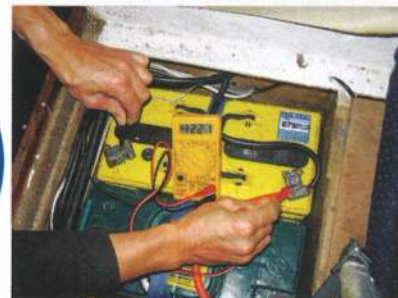
Using a digital multimeter to check battery voltage. At 12.21V this is half discharged and needs to be recharged to avoid shortening its lifespan
