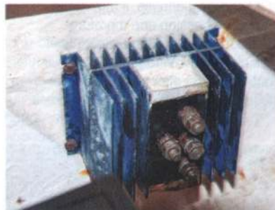
A split charge diode set that has seen better days and is ripe for replacement
