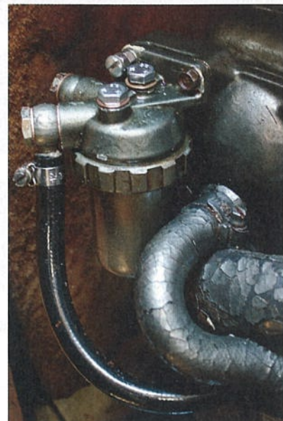
Don't forget the secondary fuel filter on the engine. If the primary filter has been clogged this one might be too.
