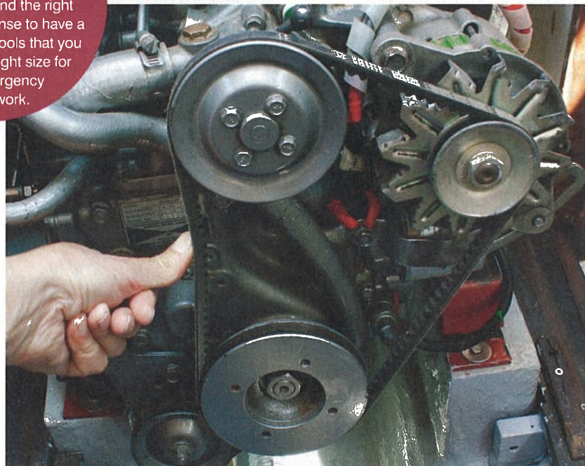
Check condition and tension of the alternator drive belt. For correct tension there should be some deflection like this, but no more than 1/2 in (13mm)
