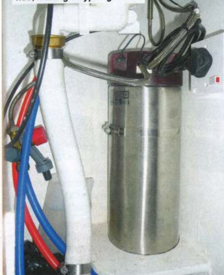
Due to the serious battery capacity and inverter on board it was possible to fit an instant boiling water tank and induction hob, making Calypso gas-free
