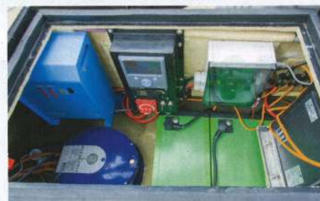
Motor, inverter, regulator and wiring can all fit into a fairly small space where a diesel would have been
