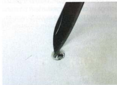
5 Lightly abrade the area around the holes with 240-grit paper and then ream the edges with a knife. This helps ensure maximum adhesion of the gelcoat filler. Clean out all swarf.
