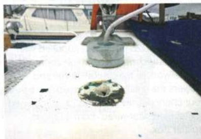
2 This was the location of an old cable deck gland. First clean the area thoroughly, in particular make sure all the old sealant is removed.
