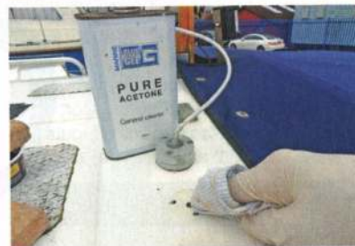
3 Use a solvent to ensure a grease-free surface and also keep the holes dry to ensure good adhesion when you come to fit the patch underneath.
