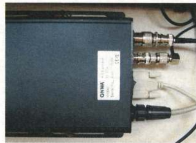
The unit in place screwed to the bulkhead above the chart table. From the top the connections are: VHF, GPS, RS232 serial and power. You can see I needed to juggle with some adaptors for the radio and GPS feeds, luckily these are easily come by
