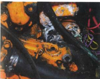
With the alternator removed the salt water leak from the heat exchanger is revealed
