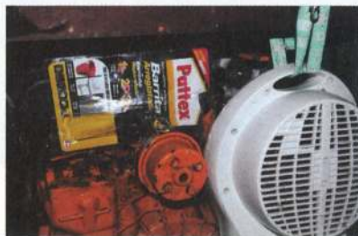
Repairing the hole with two part epoxy putty and Sikaflex at Camarindas
