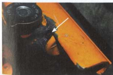
Finger pressure over the corroded area of the heat exchanger led to a big hole
